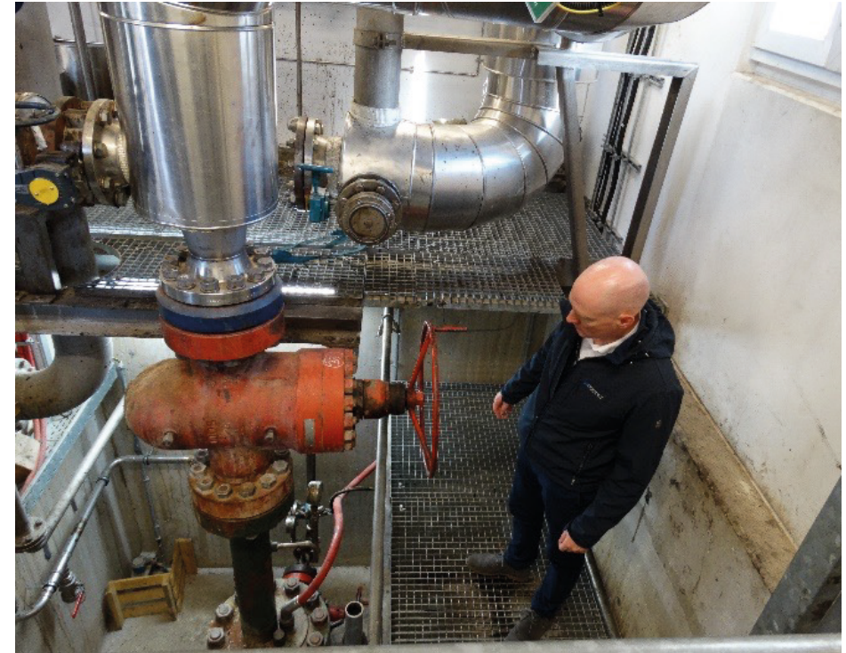
Viewing a deep geothermal well
